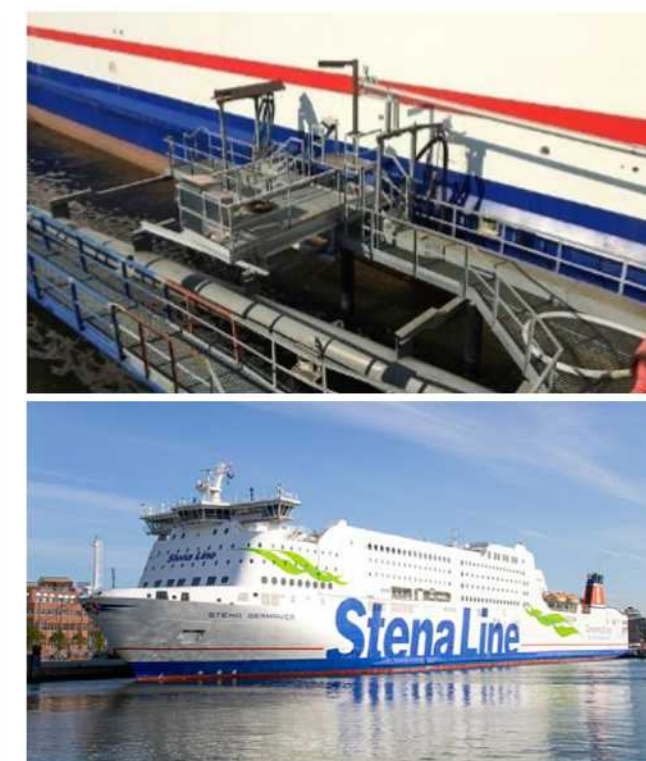
Figure 5 - Stena Germanica Methanol Refuelling Infrastructure
